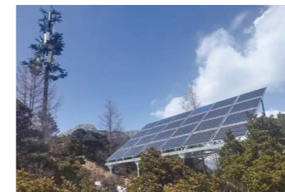
Telecom base applicaiton
