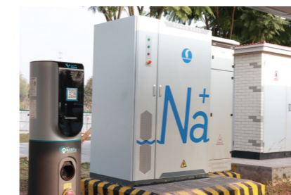
NaESS+PV+Charger Integration Project
